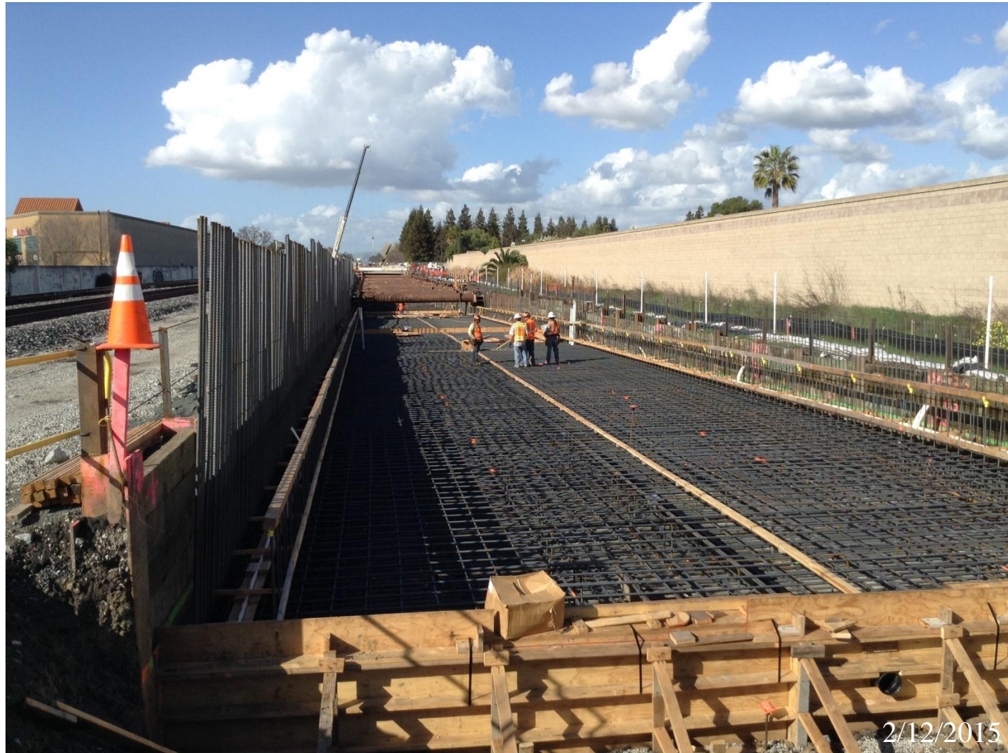
Reinforcing at the southern end of the trench at Dixon Landing Road in Milpitas
