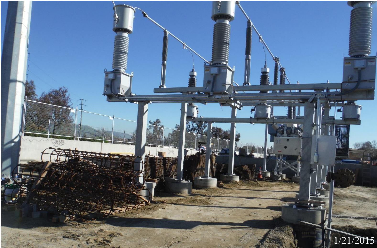
Substation grading and compaction at the wayside facility at Railroad Court, south of Abel Street, in the City of Milpitas
