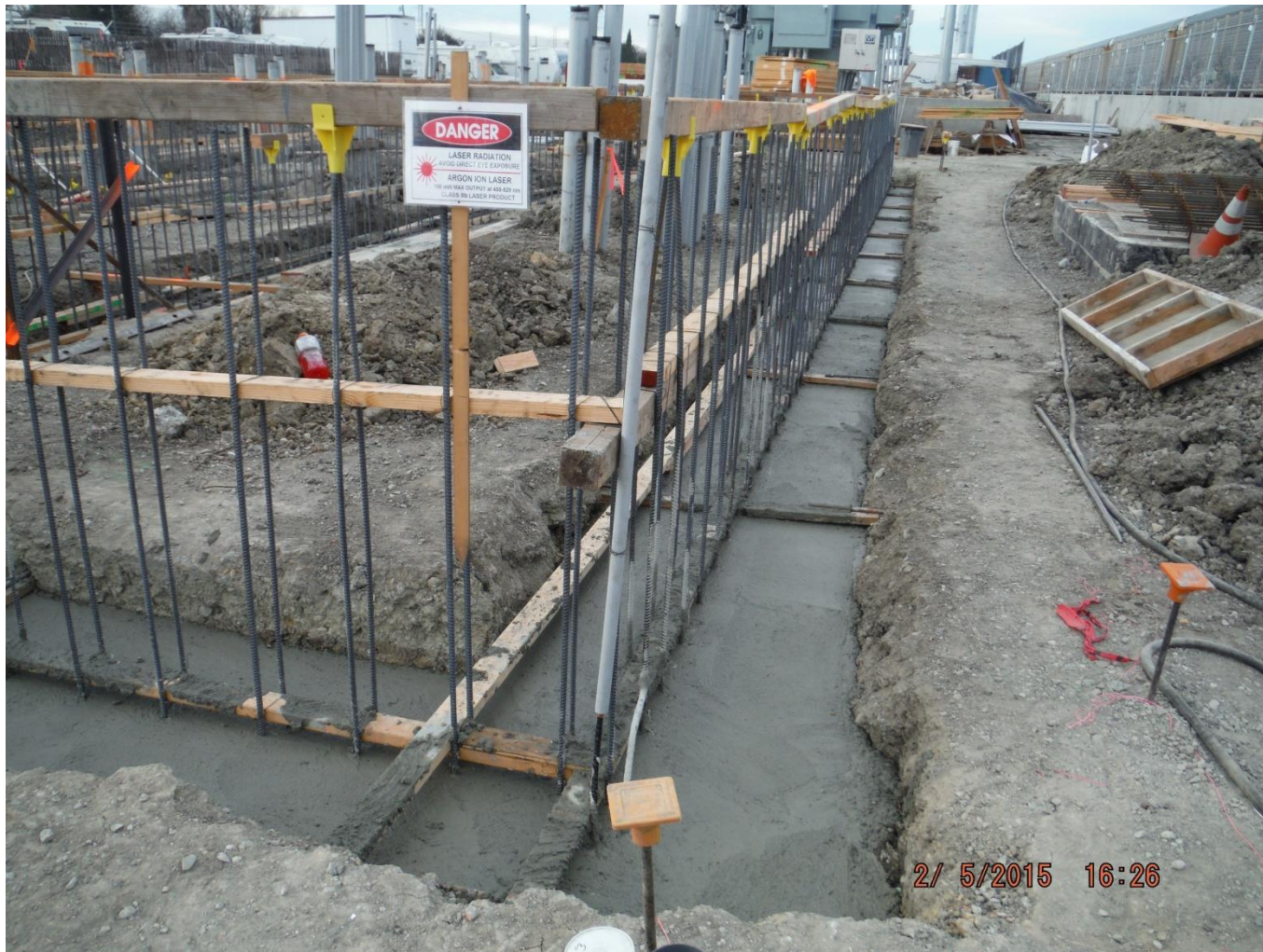
Wayside facility foundation pour at Railroad Court, south of Abel Street in the City of Milpitas
