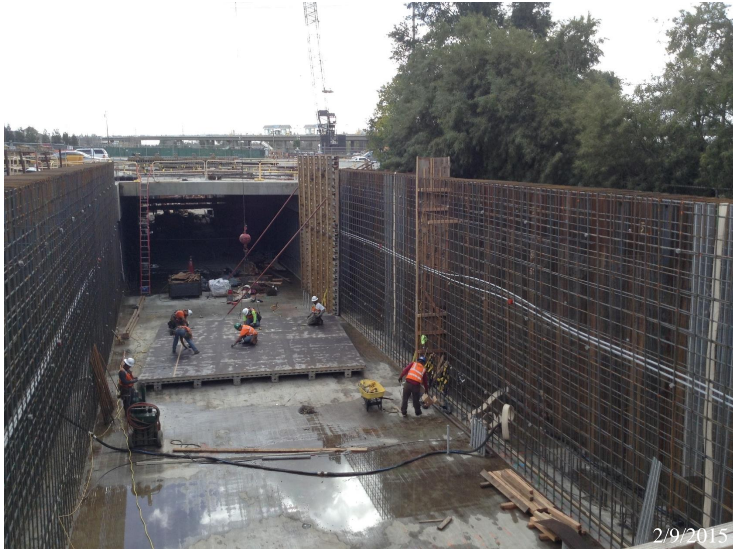
Rebar and formwork for the Milpitas trench walls south of Montague Expressway in the city of Milpitas
