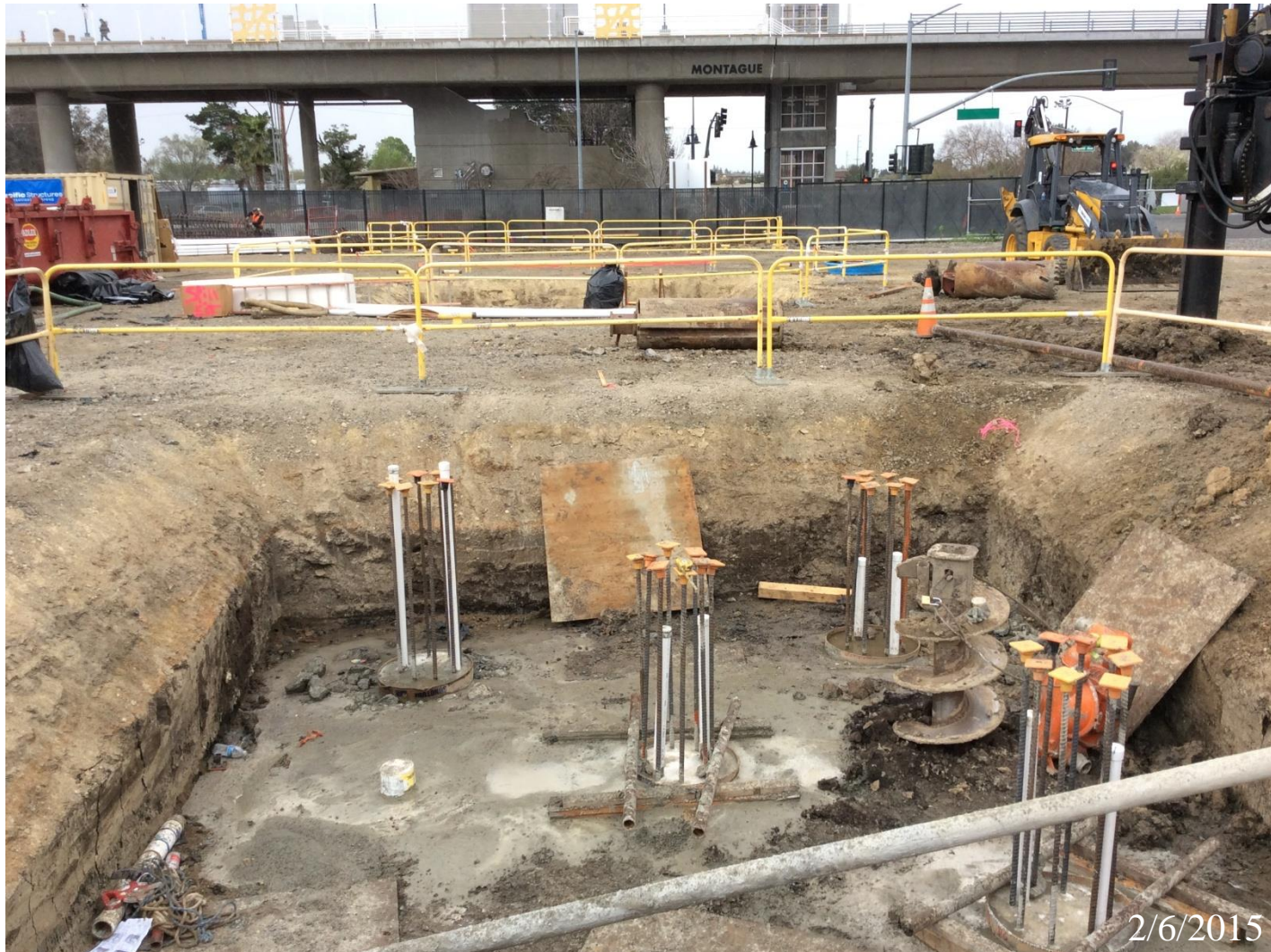
Foundation for the Pedestrian Overcrossing from the Milpitas Station to the Montague LRT Station
