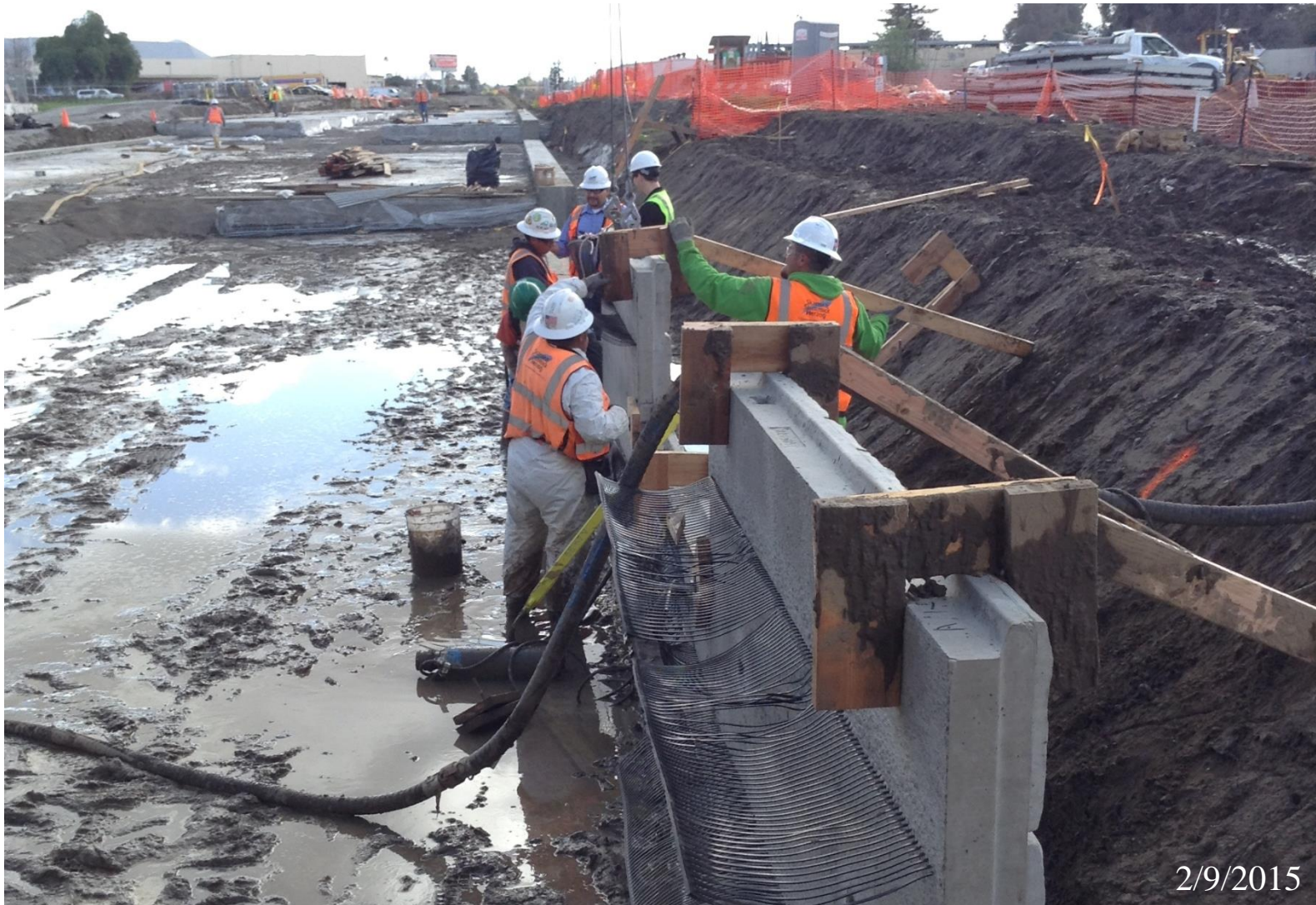
Installing Mechanically-Stabilized Earth (MSE) walls along the aerial structure south of Berryessa Station
