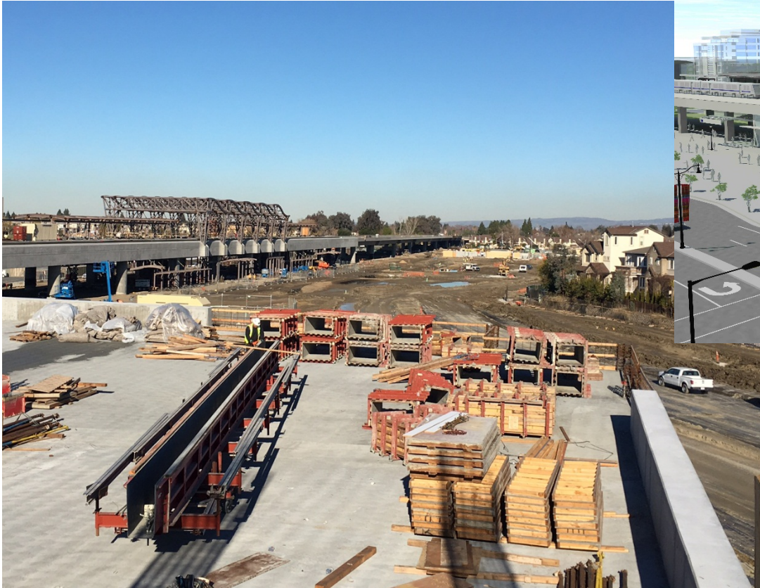
View of the Berryessa Station taking shape from the third floor of the parking structure.
